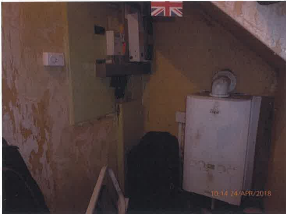
Boiler and carbon monoxide detector
