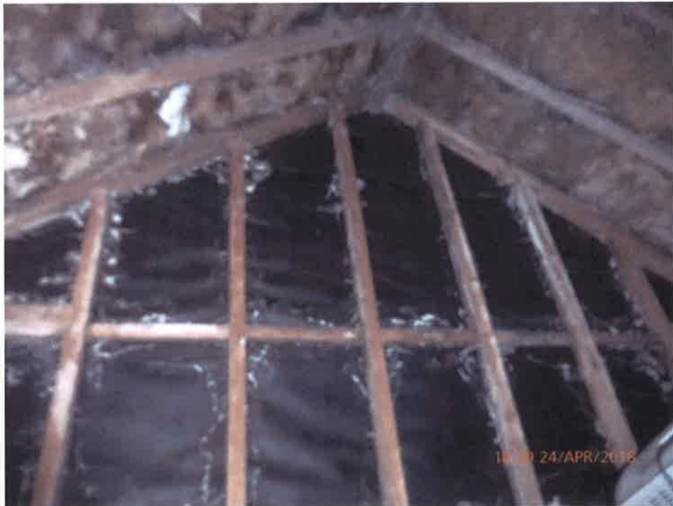
Dampness in the roof space
