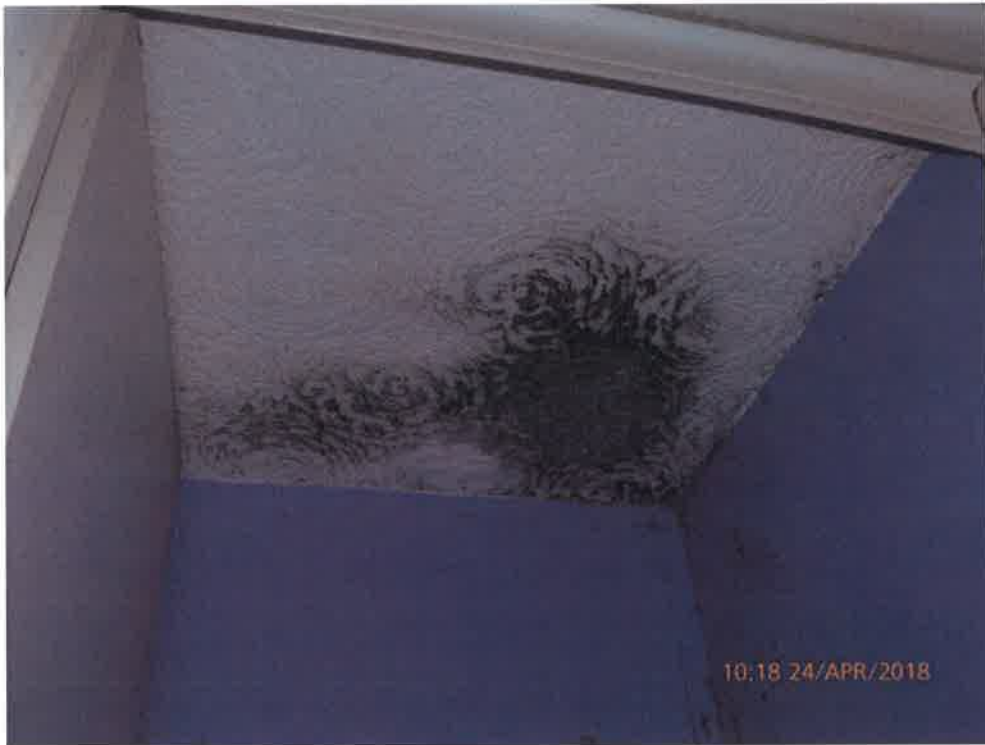
Mould on ceiling of the first floor
