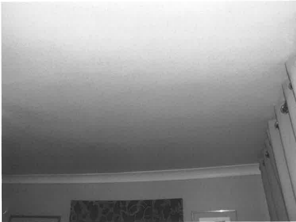
Living Room Ceiling (No Smoke Detector)
