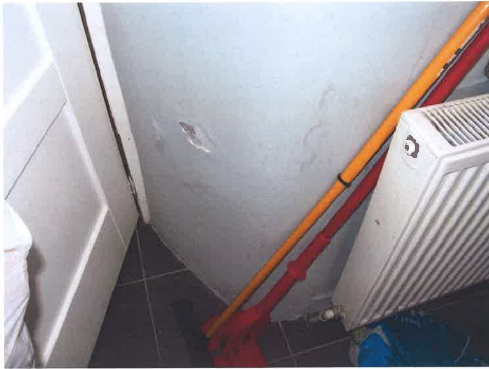
Dampness in Kitchen (1)
