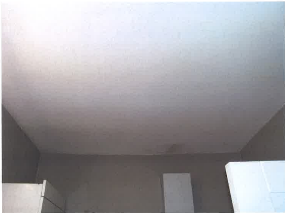
Kitchen Ceiling (No Heat Detector)
