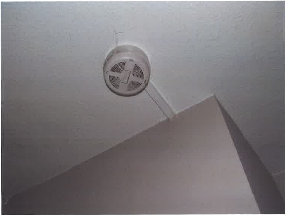
Hall Smoke Detector
