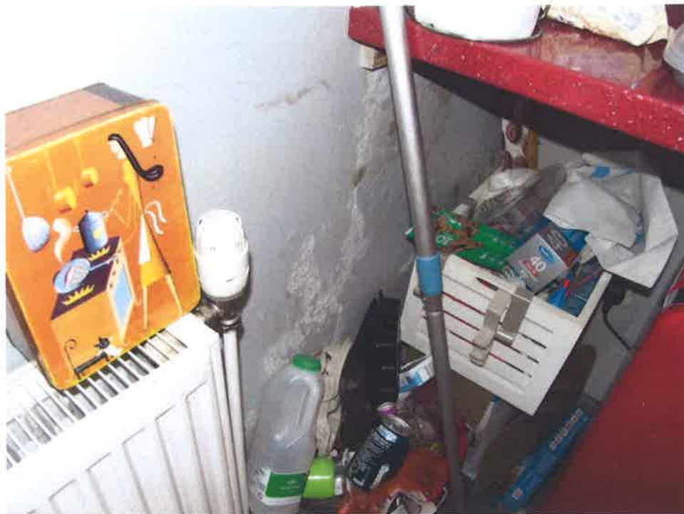
Dampness in Kitchen (2)
