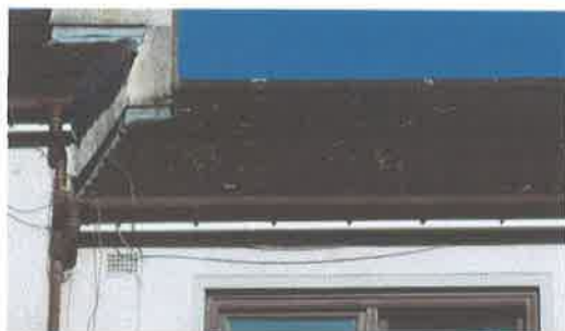
Photo 13 – Blocked gutters to front
