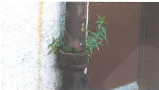
Photo 12 – Vegetation on rear downpipe
