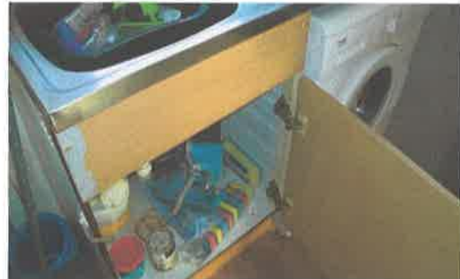
Photo 3 – Damaged kitchen unit
