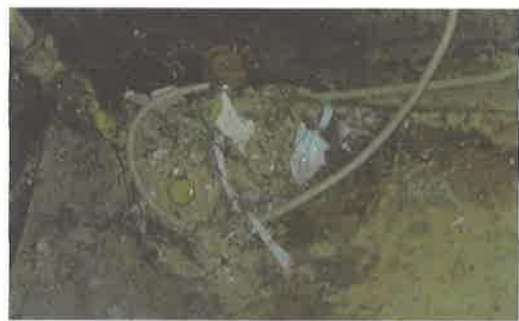
Photo 5 – Exposed area next to sink
