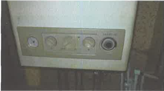
Photo 2 – Gas boiler in landing cupboard
