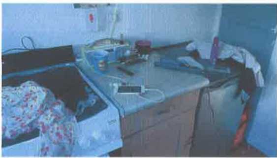
Photo 4 – Kitchen unit with damaged door
