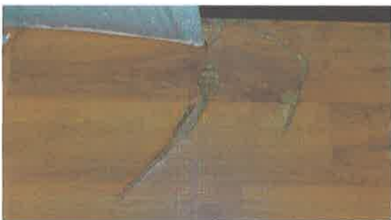
Photo 6 – Damaged kitchen floor surface
