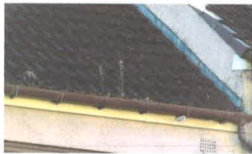
Photo – 11 Blocked gutters to rear
