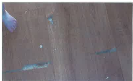
Photo 7 – Damaged kitchen floor surface
