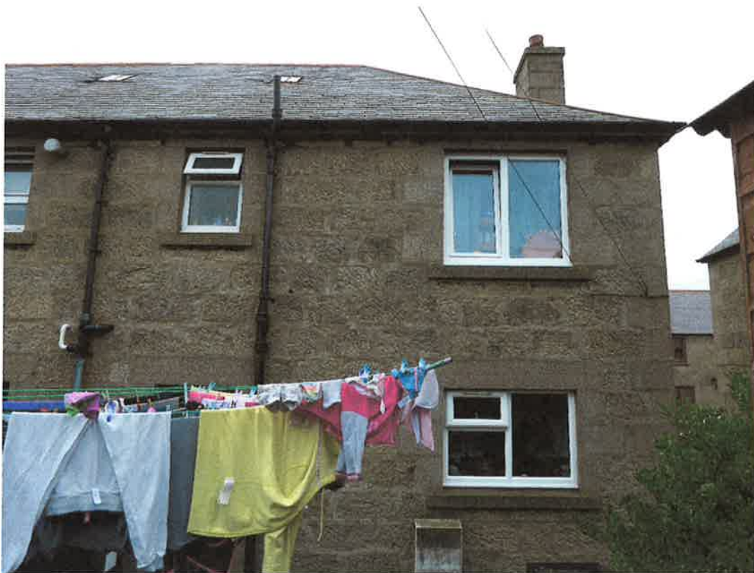
Rear elevation – new 1 st floor bedroom window tilted inwards.
