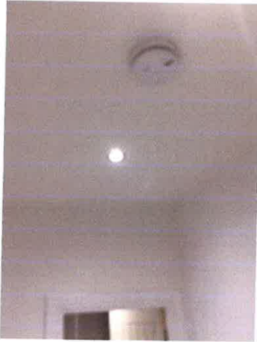
Photograph 3 – Hall: smoke detector
