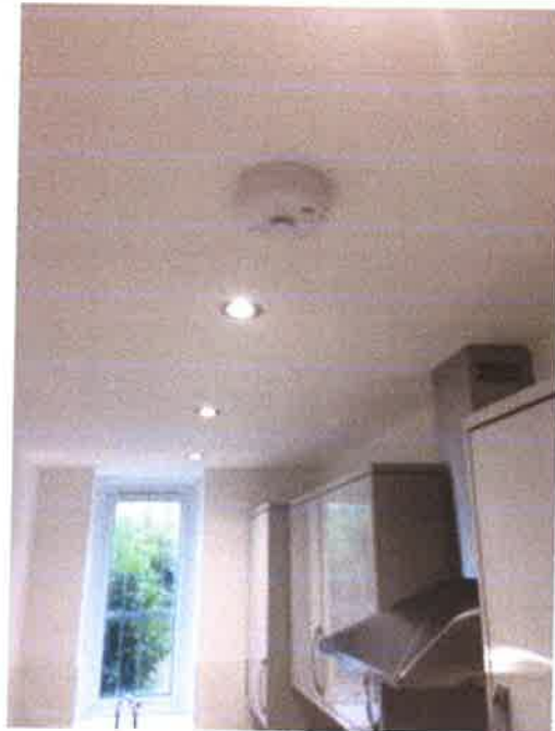
Photograph 4 –Kitchen: heat detector
