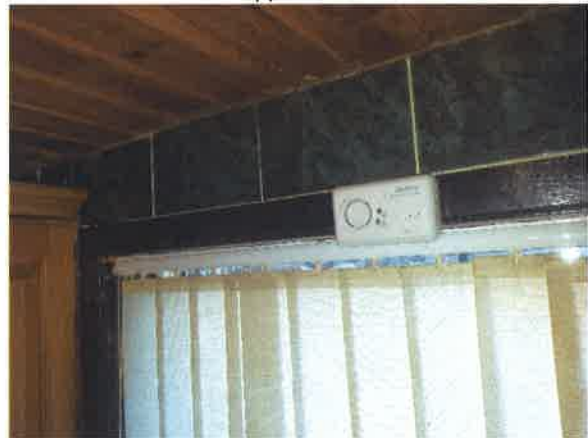
18 Carbon Monoxide detector in Kitchen above window.
