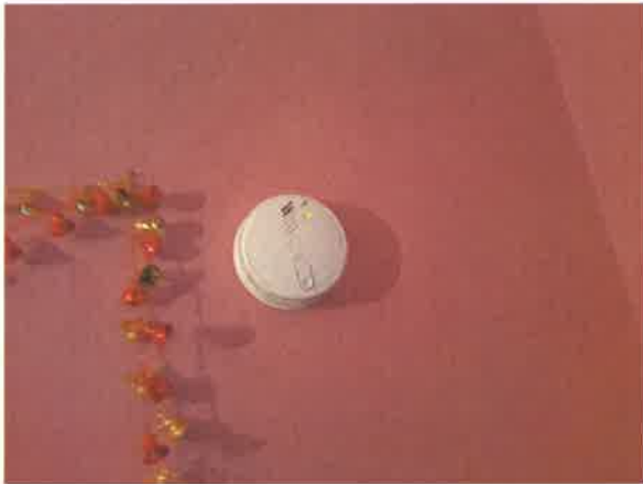
13 Smoke Detector in Living Room (rear)
