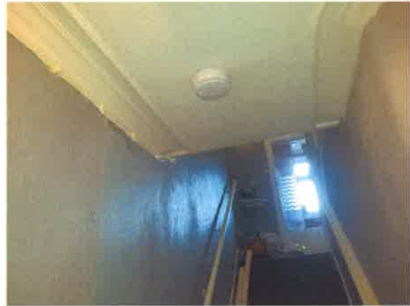
14 Smoke Detector in ground floor hall.
