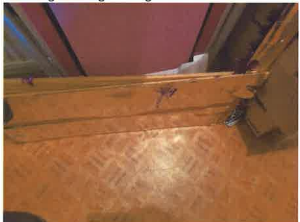
30 Stair gate and builders debris.
