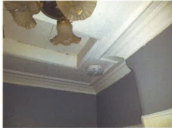
16 Smoke detector in upper hall.
