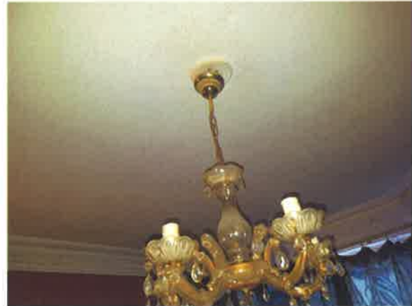
12 Front Living Room – loose light fitting to ceiling.
