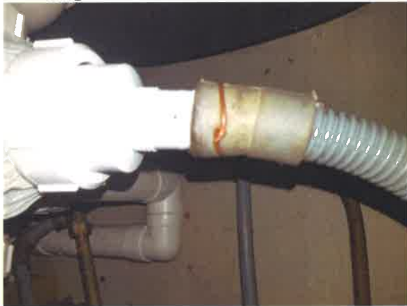
21 Inappropriate plumbing connection with copper wire in lieu of jubilee clip.
