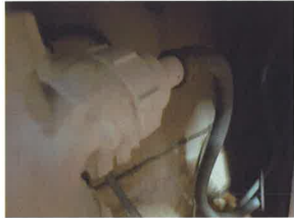
22 Material within plumbing connection affecting seal.
