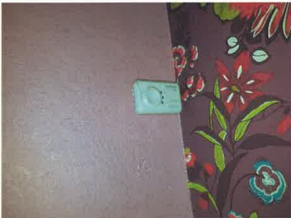
17 Carbon Monoxide detector in rear Living Room.
