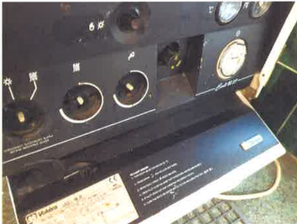
19 Missing thumb turn controls to boiler.
