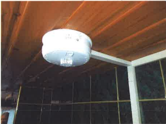
15 Heat detector in Kitchen.
