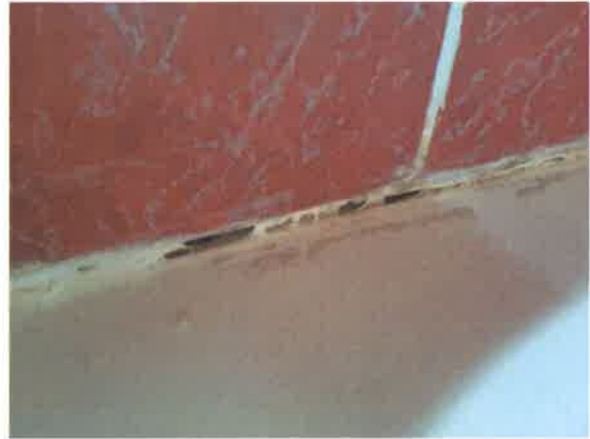
2 Close view of defective bathroom sealant.
