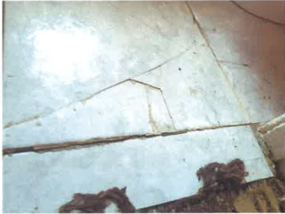
7 Close view of defective, loose and raised bathroom floor tiles at threshold
