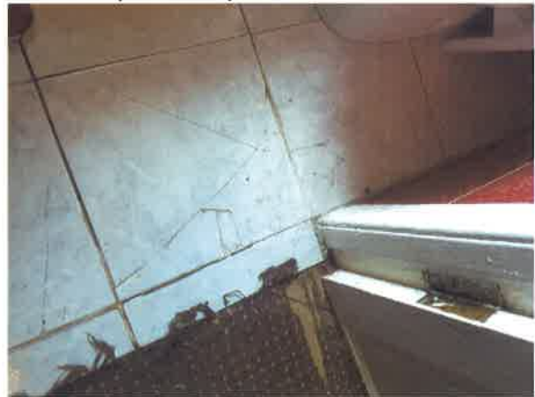
6 Cracked and defective bathroom floor tiling.
