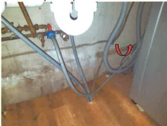
23 Loose pipework – no clipping. Pipework looped and not correctly fitted.
