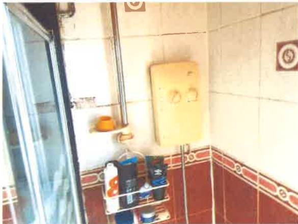
9 Electric shower – operational and producing hot water on testing.
