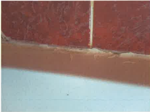
3 Close view of defective bathroom sealant.
