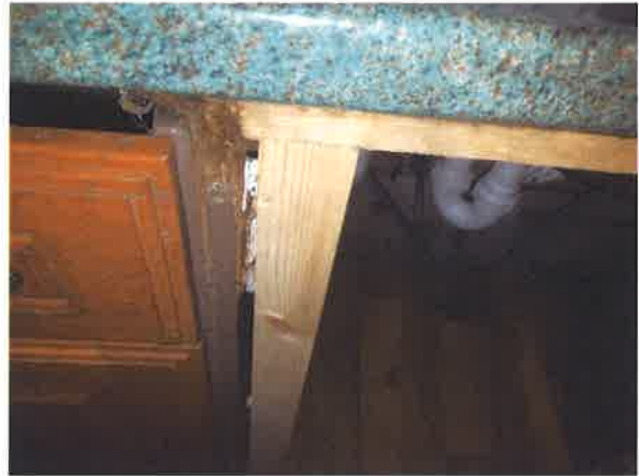
26 Damaged kitchen units.
