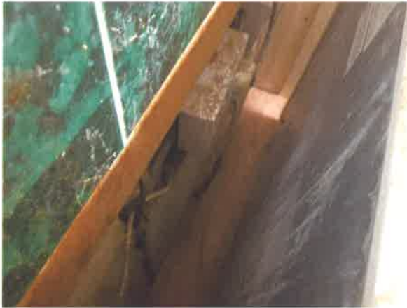
25 Poor electrics behind chest freezer, backplate not secured.
