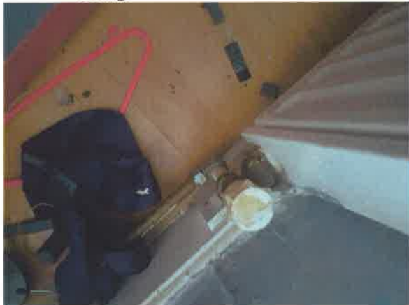
11 Ciaran's Bedroom – socket located behind radiator pipework.
