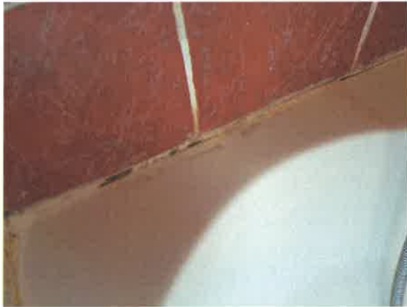
1 View of bathroom sealant.
