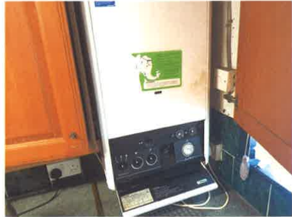
20 General view of boiler – unable to be tested.
