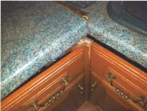
27 Damaged kitchen units.
