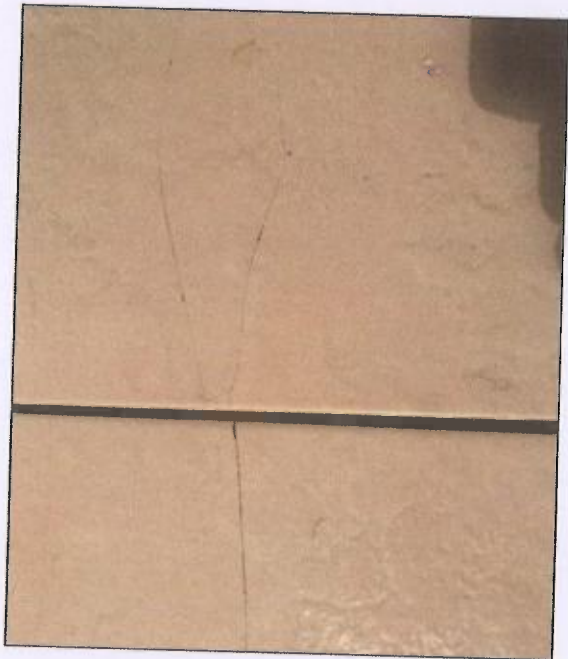
Ceramic floor tiles have evidence of surface cracking
