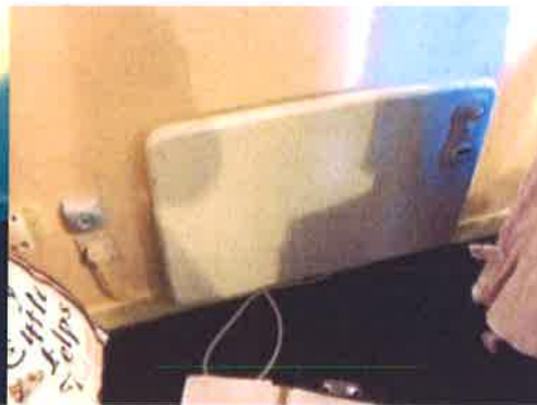
Electric panel heater – living room 13 September 2016
