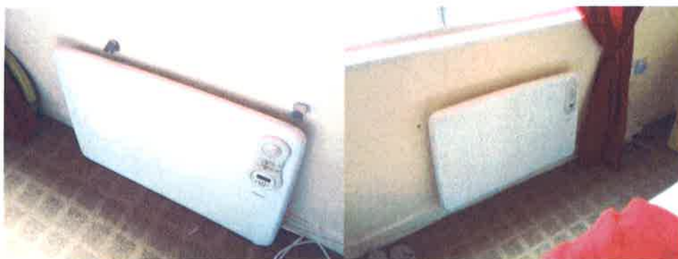
Electric panel heater – bedroom 20 June 2016
