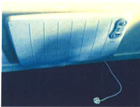
Electric panel heater – living room 20 June 2016
