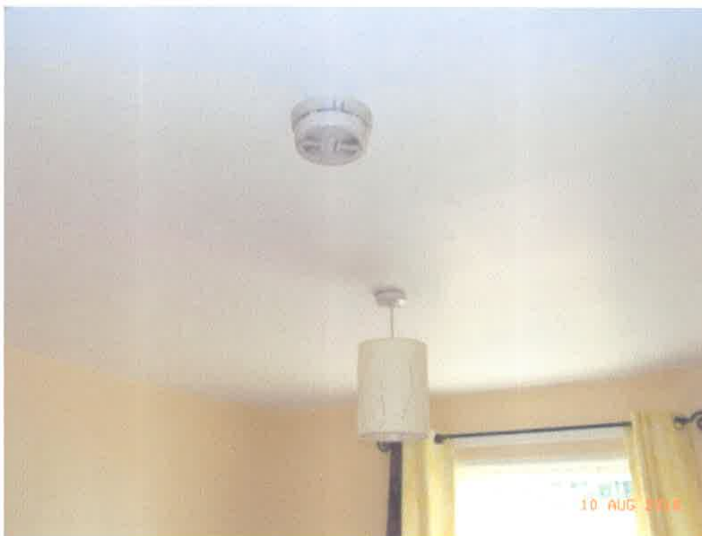
Bedroom 1 smoke detector
