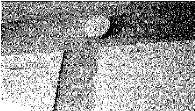
Photo 8: CO2 alarm fitted outside boiler cupboard
