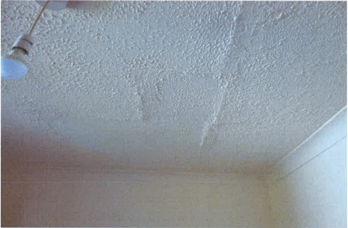
Lounge ceiling – Recent patch repair
