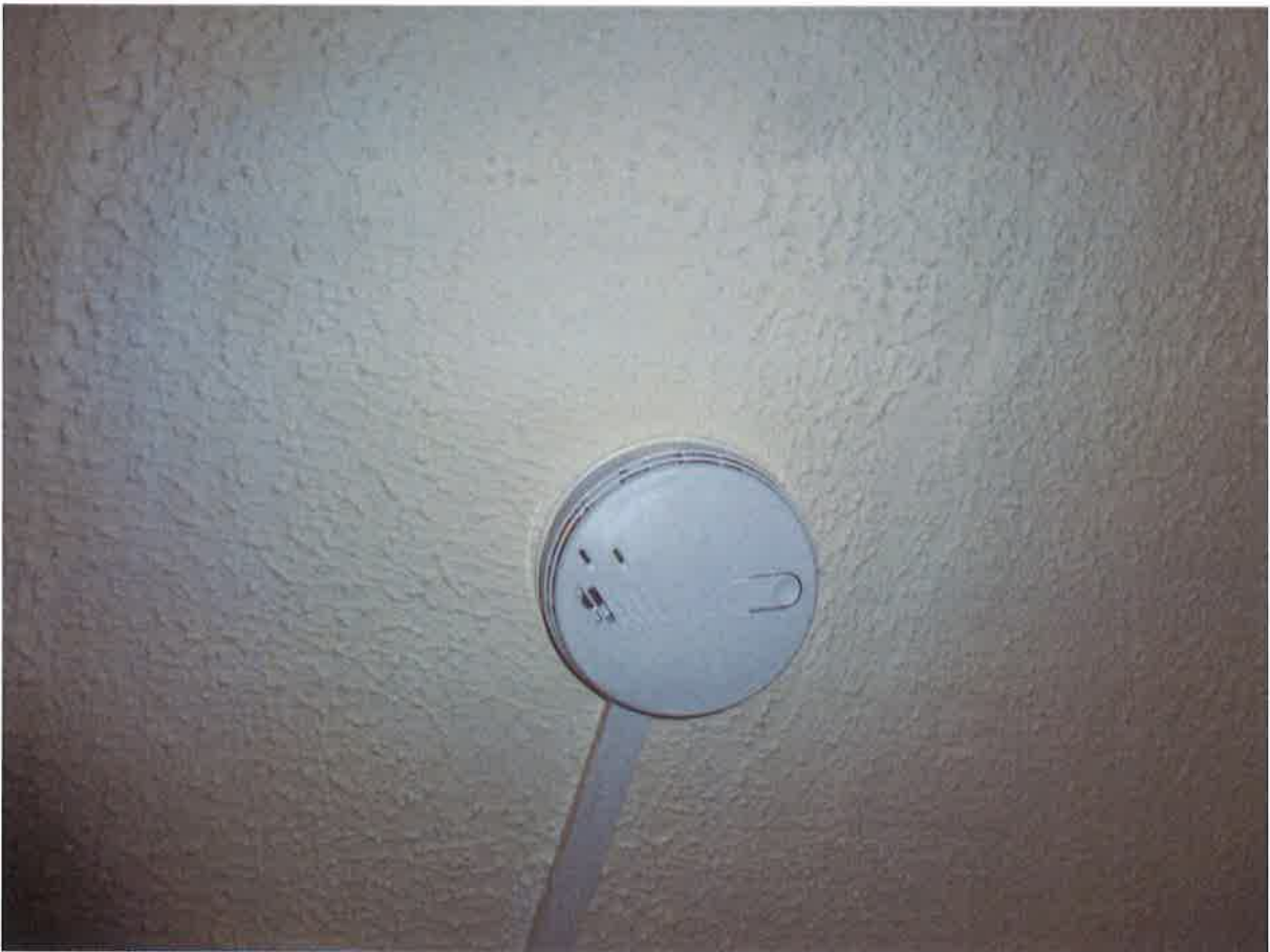
Operating Smoke alarm
