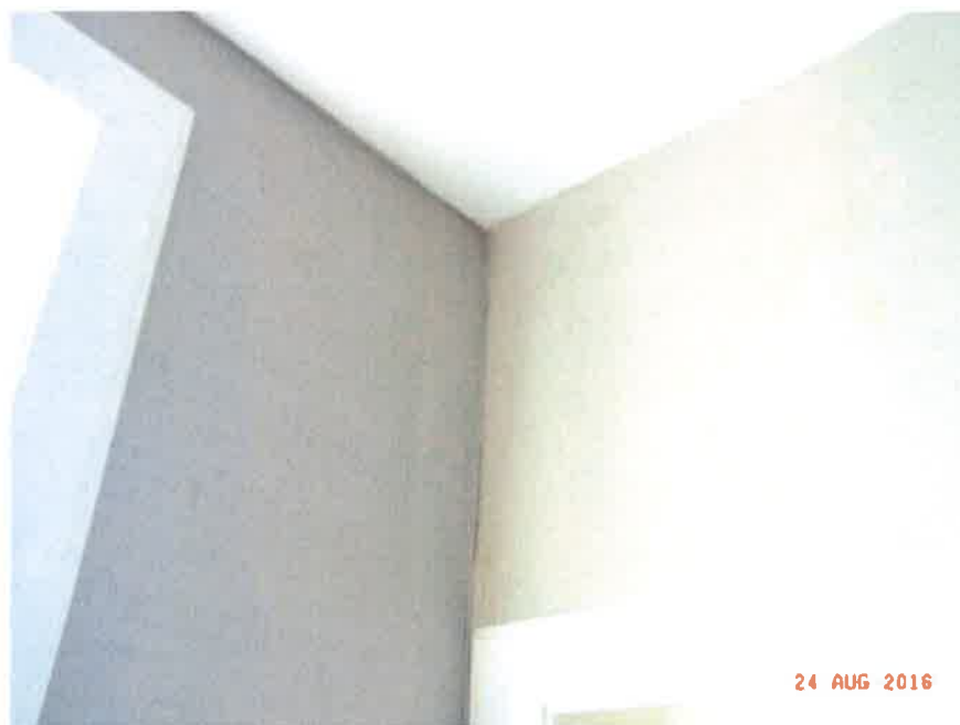
Kitchen/Dining Room (Room south east) – Upper wall/ceiling
