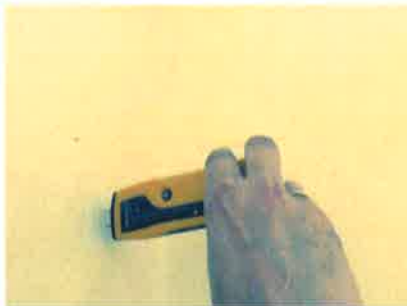
Damp meter reading – rear bedroom (right hand wall)
