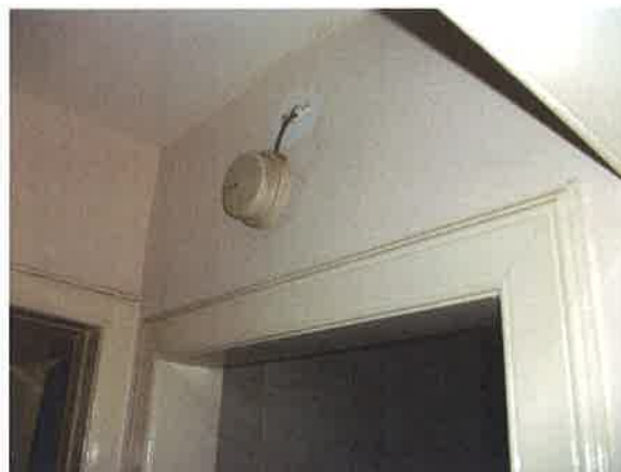
02 - Hall - smoke detector (not working at inspection)
