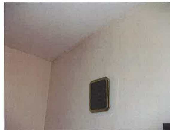
06 - Lounge - dampness at ceiling south gable wall (visible damp stains but not tested or measured at inspection as furniture prevented access)
