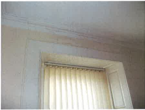
07 - Front bedroom - dampness above window (Front gutter is directly above the window)
