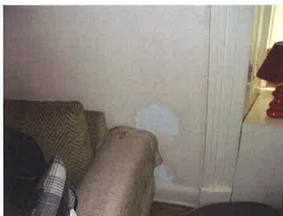
04 - Lounge - dampness at south gable window (severe dampness levels recorded at inspection)
