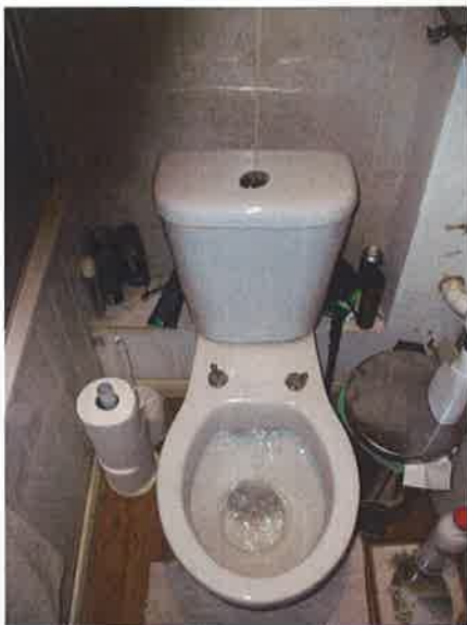
09 - WC - no seat (and flush mechanism malfunction)
