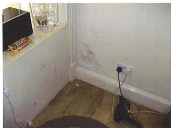
05 - Lounge - dampness at SW corner (severe dampness levels recorded at inspection)
