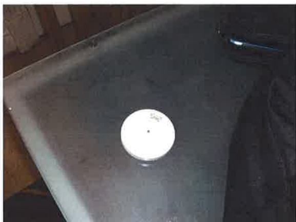
03 - Lounge - battery-operated smoke alarm (loose unit but working at inspection)
