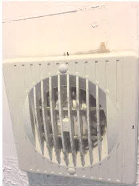
Bathroom extractor fan-vanes with dust
