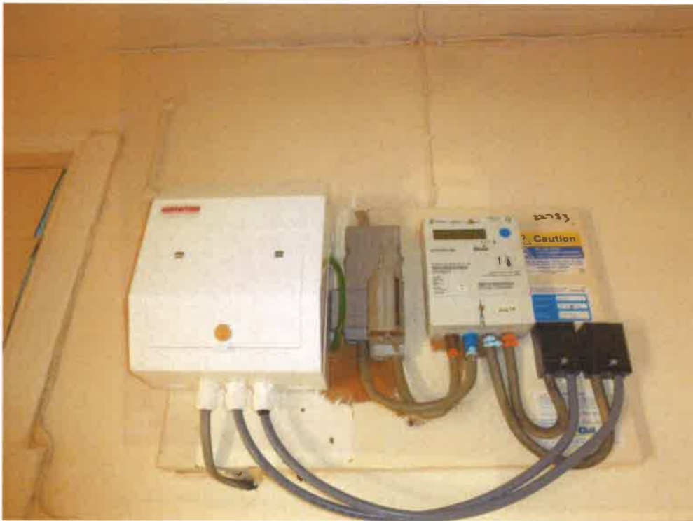
New distribution board
