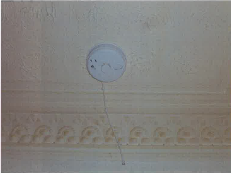
Lounge smoke detector
