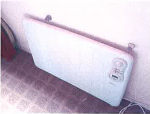
Bedroom – electric panel heater
