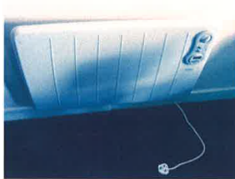
Living room – electric panel heater
