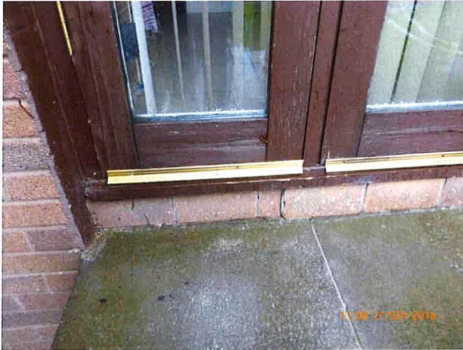
Detail of door showing fungal growth
