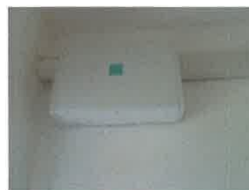
10. Recently fitted ventilation unit
