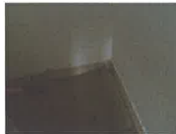
7. Mould at bedroom skirting
