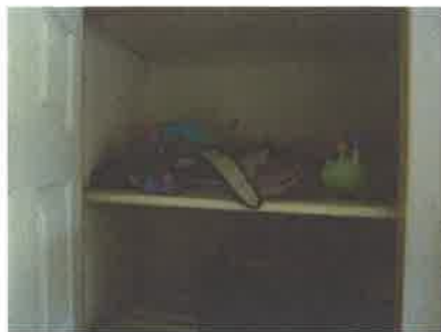
6. Hall cupboard showing mould growth
