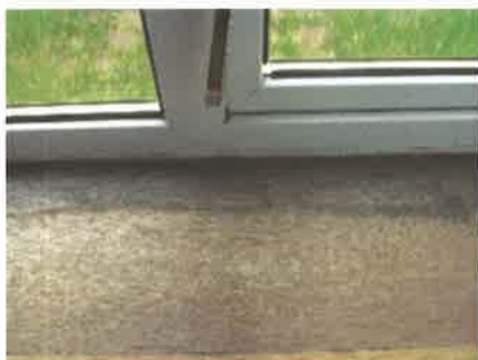
8. Mould/staining window cill
