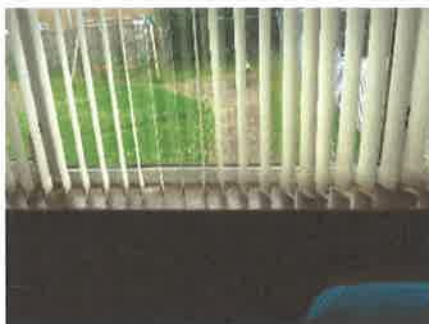
9. Mould to living room blind
