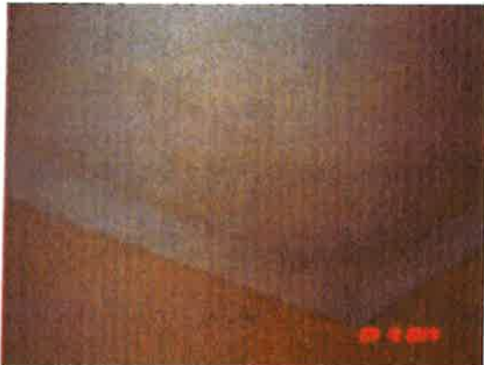
Cracking in Dining Room ceiling
