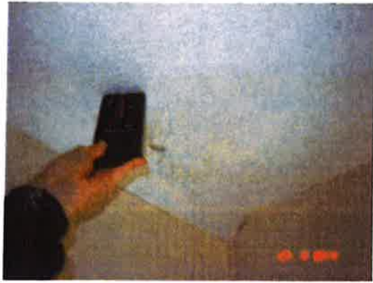
Stain at entrance stair ceiling
