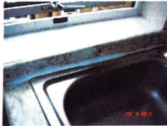
Repair at worktop
