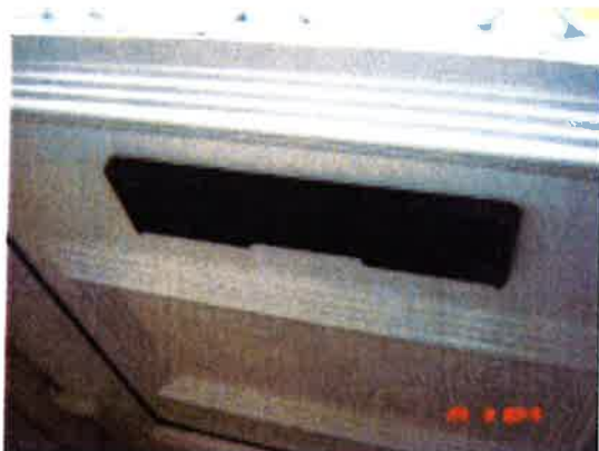
Missing inner flap at letter box
