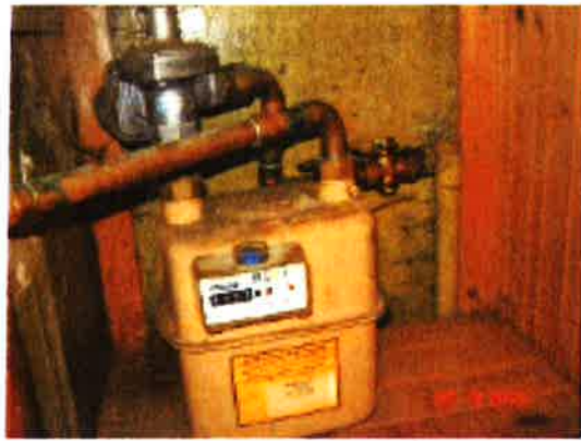
Old staining at Hall cupboard
