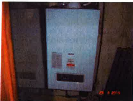
New central heating boiler
