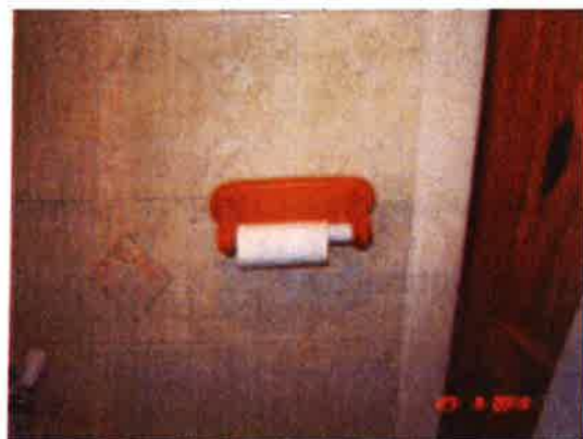
Loose fitting toilet roll holder
