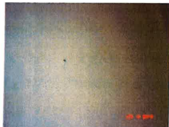
Small holes in DR wall.
