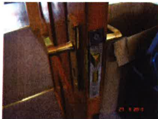
New door handle/lock in bedroom 1
