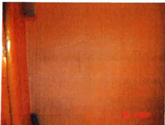
Loose wallpaper in Hall.
