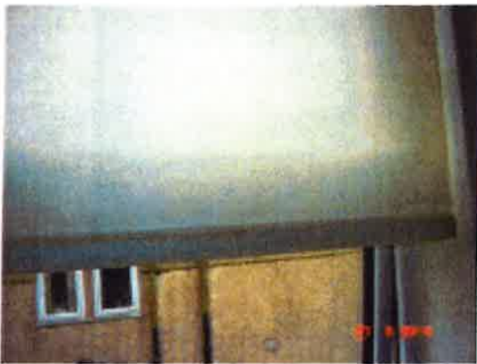
Kitchen blind-some staining
