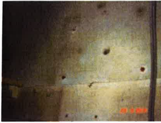
Holes in Bedroom 1 cupboard
