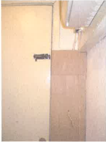
ENTRANCE DOOR FRAME/WIRING FOR DOOR BUZZER
