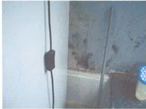
KITCHEN WALL- MOULD
