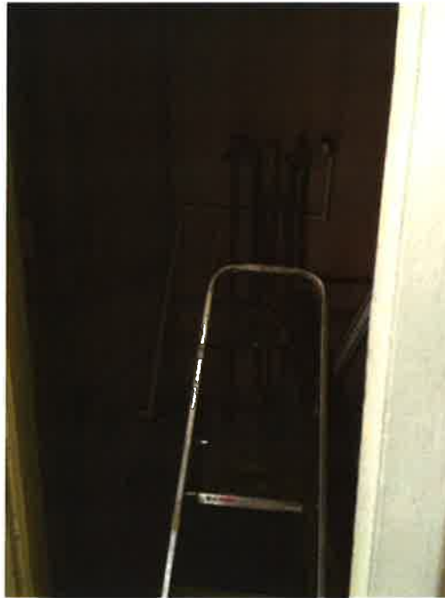
Boiler cupboard (hallway)
