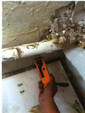
Damp meter reading – internal wall – washing machine space
