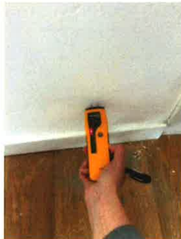
Damp meter reading – external wall - near back door
