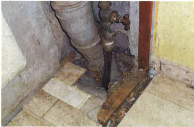
03 - Kitchen (gap behind appliance)
