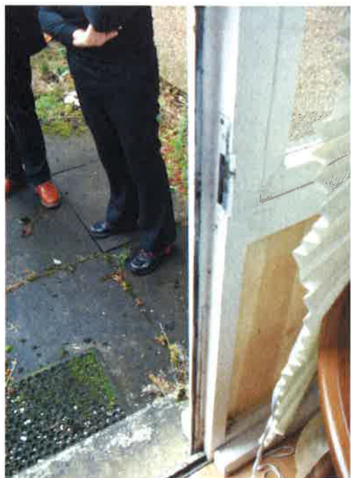
06 - Rear door (damaged seal)
