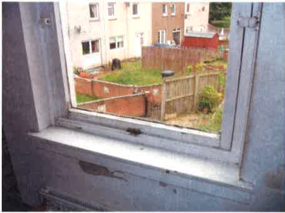
07 - Bedroom window – missing handle
