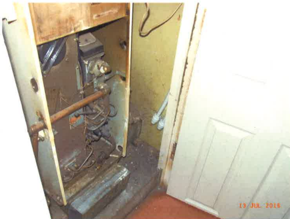
Redundant central heating boiler and replacement cupboard door
